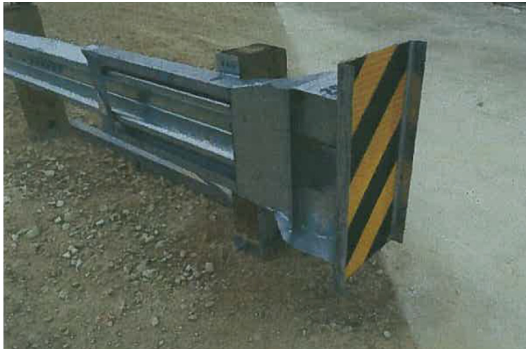
ET-Plus as installed. ROA.11685.
